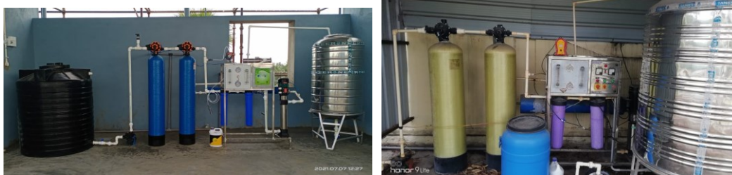
Reverse Osmosis Plant
